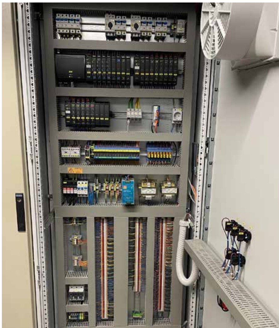
Control cabinet in Germany's largest BACnet/SC-based property © Tino Erler, SI-Building Automation
